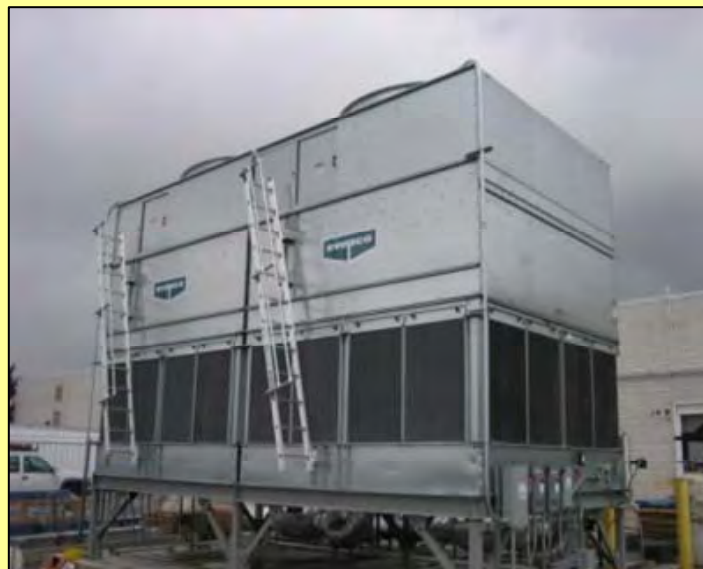
High efficiency cooling towers at Ogden manufacturing plant (credit: ETC Group, LLC)
