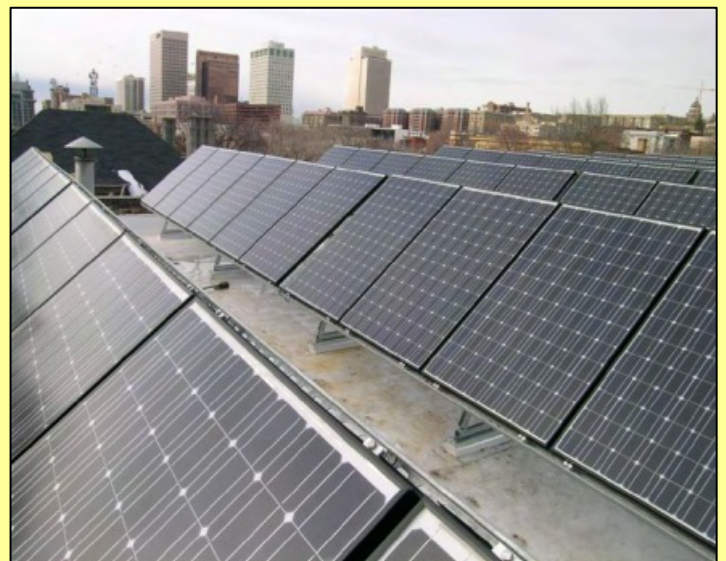
Solar PV units on roof of Ashby Apartments in Salt Lake City (credit: LaPorte Group)
