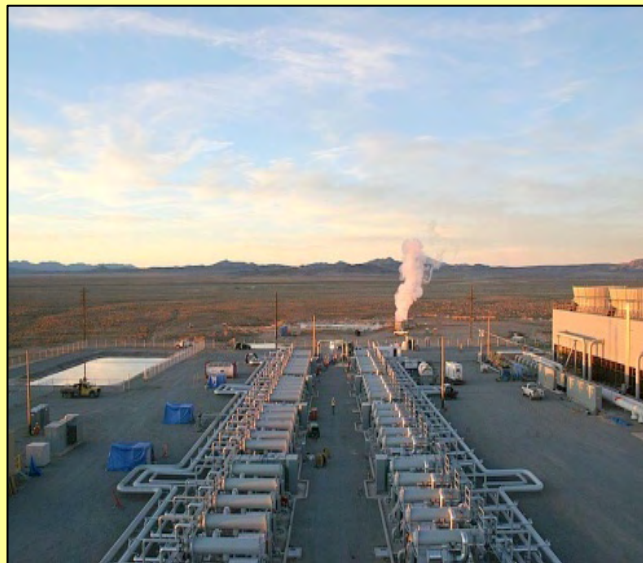
Raser Technologies' Thermo Power Plant in Beaver County, Utah.
