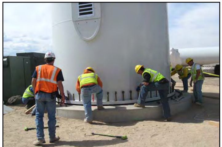
Workers finalize the installation of the first wind turbine base at the Milford Wind Farm located in Milford, Utah.
