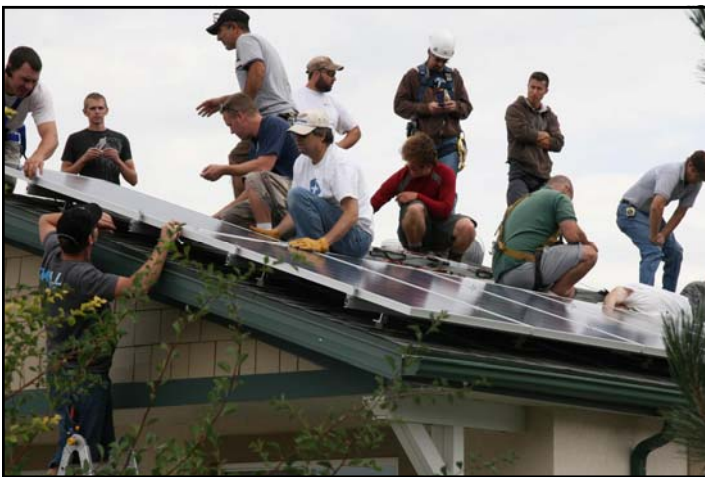
Salt Lake Community College students help install solar panels at a low income house in Kearns, Utah as part of a PV Solar training course at the College.
