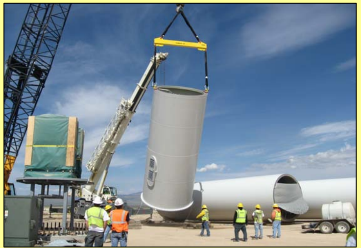
Wind turbine towers at the Milford Wind Project construction zone (credit: First Wind)
