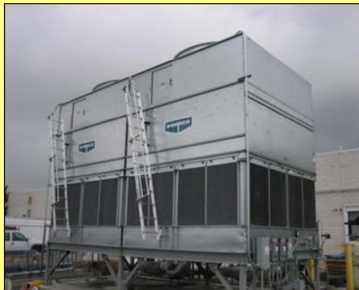
High efficiency cooling towers at Ogden manufacturing plant (credit: ETC Group, LLC)
