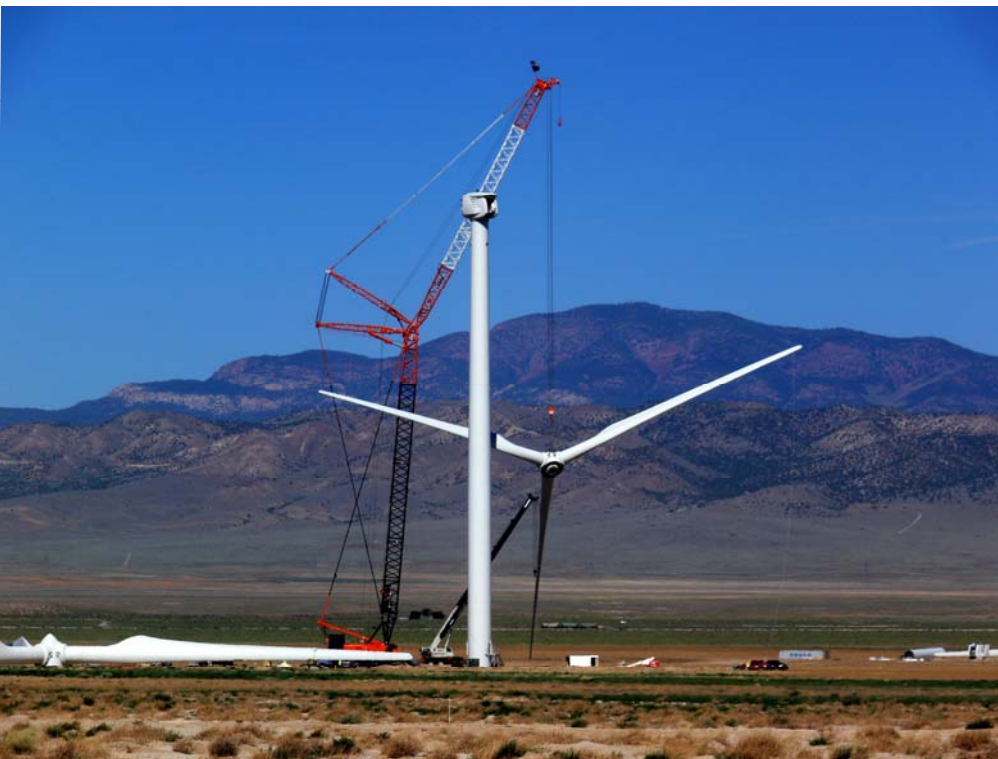
A massive wind turbine is lifted for installation at the Milford Wind Farm construction site. This wind project will be the largest renewable energy facility in Utah.
