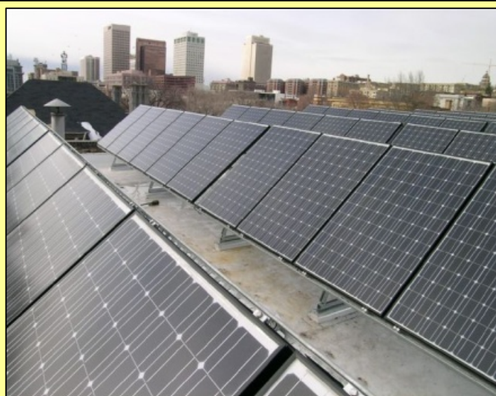
Solar PV units on roof of Ashby Apartments in Salt Lake City (credit: LaPorte Group)
