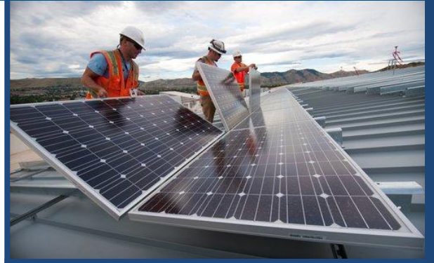
Installers should be properly licensed and familiar with all safety protocols while on the job. Credit: Dennis Schroeder, National Renewable Energy Laboratory.
