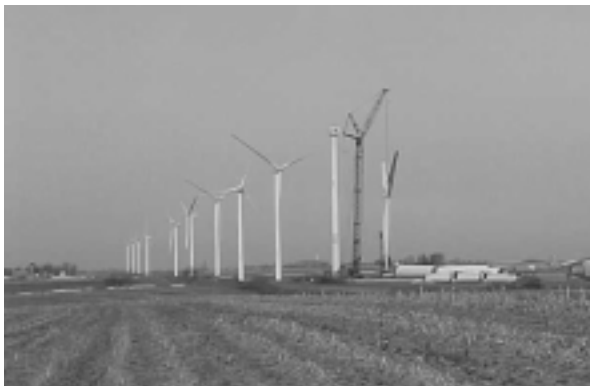
Figure 6. A large crane is used to raise a rotor into position. Photo courtesy of AWEA.
