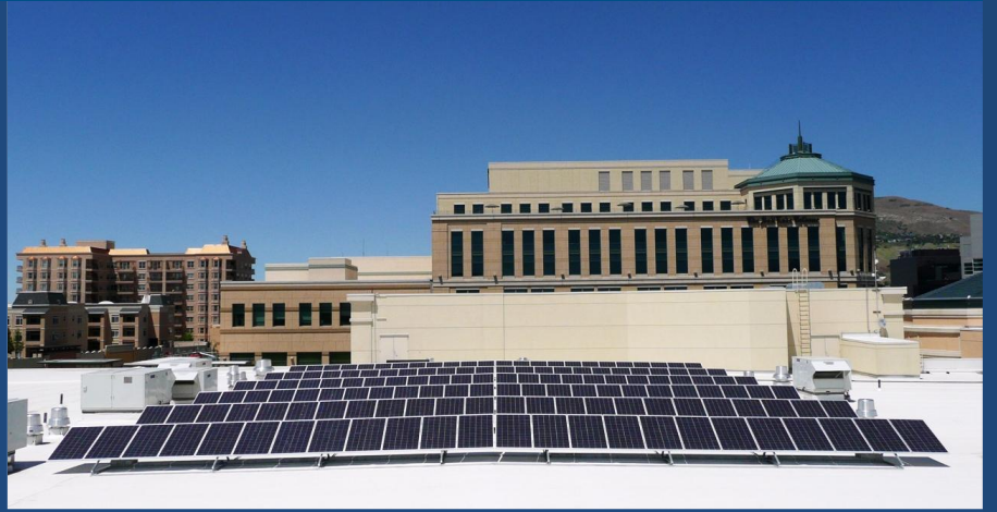
A 25-kilowatt solar photovoltaic system on the Clark Planetarium in downtown Salt Lake City. Photo Credit: Seth Jarvis.
