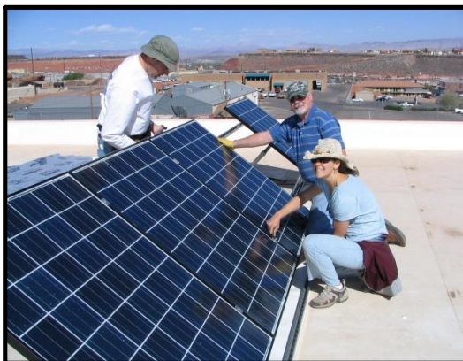
5-kW Solar PV System Installation on St. George City Power Building (Washington County) Photo Credit: Utah Clean Energy, 2007
