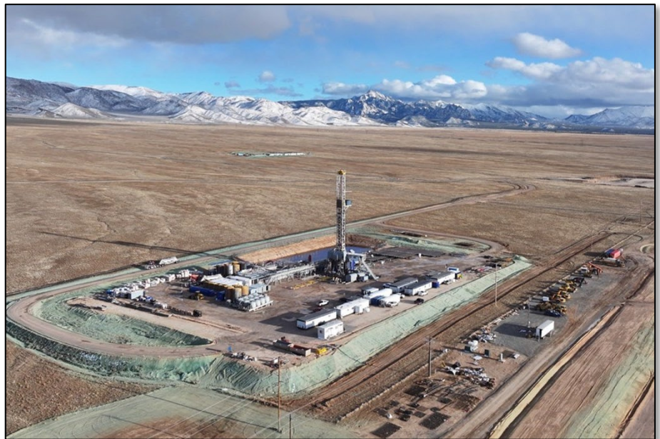
Figure 1. Fervo Energy's Cape Station Enhanced Geothermal System (EGS) Power Plant in Beaver County, Utah
